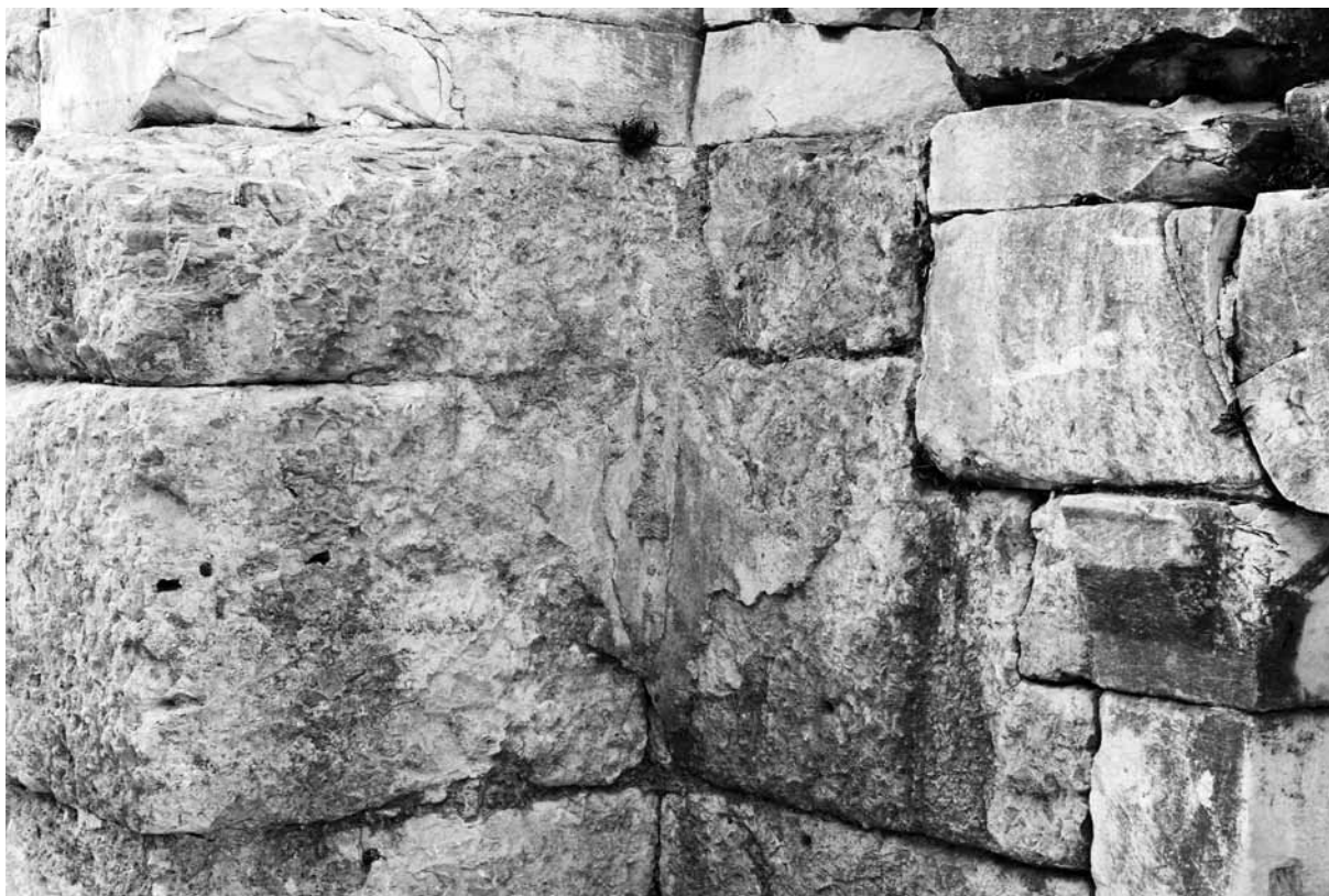
1 Traces of plaster next to SD 1
