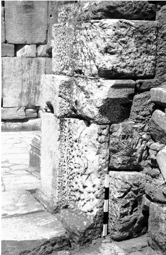
1 Original doorway in scene wall (SD 6) from south with remains of original jamb capital
